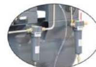
Pre Filter and After Filter
